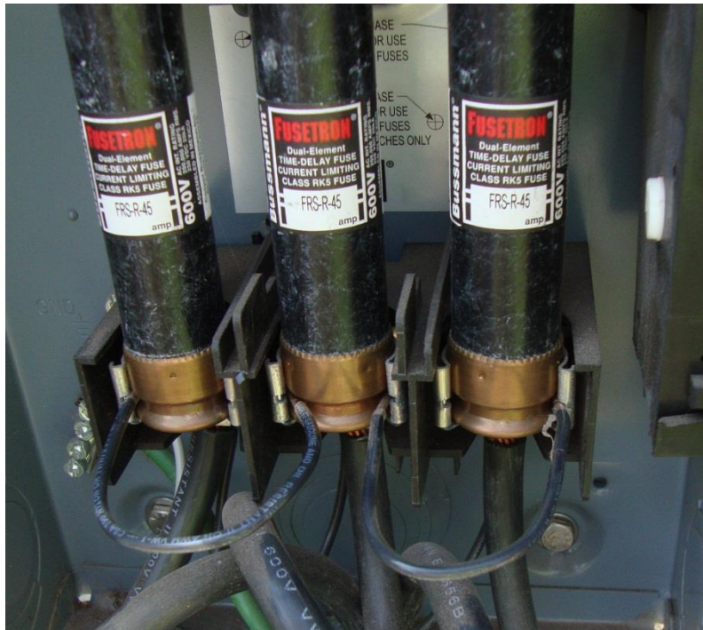
Setup for TEMPORARY shorting
